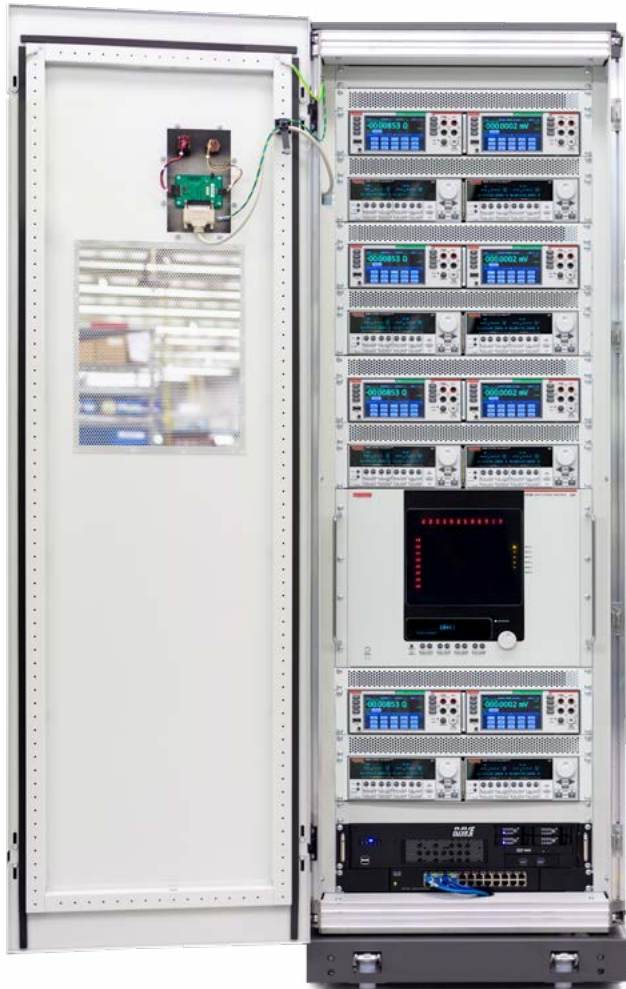
Figure 7: Typical test rack with multichannel high accuracy DMMs and related switching unit
